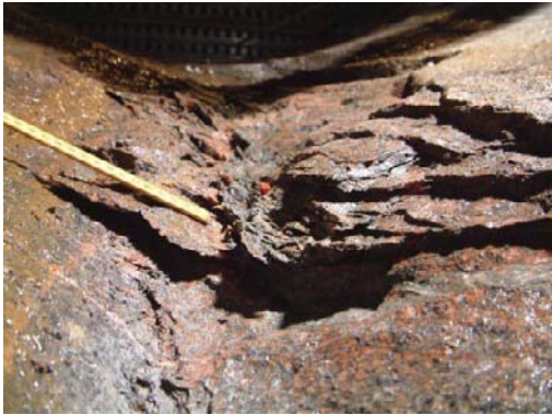
Cross section through spalled zone in the Pillar Stability Experiment (APSE) /Andersson 2007/
